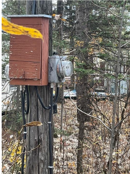
Image 5: Example Individual Power Meter
