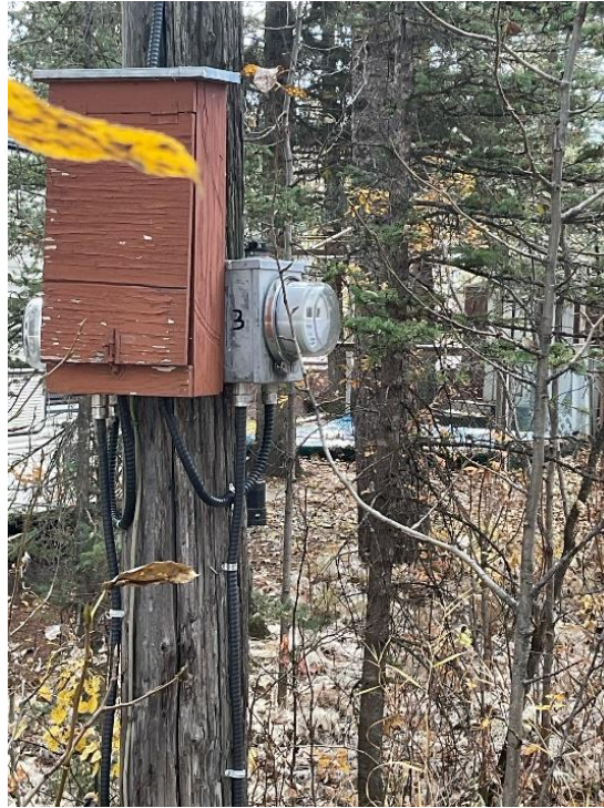
Image 5: Example Individual Power Meter
