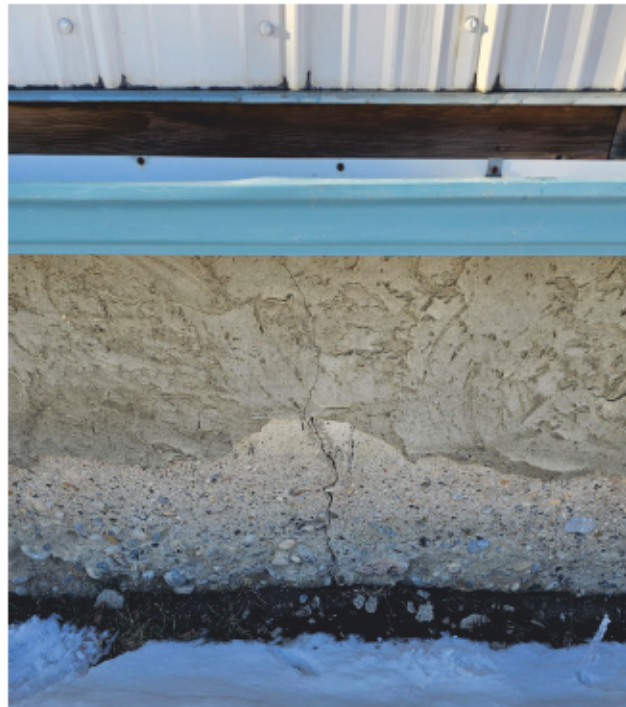
Photo 6. Foundation Cold Joints & erosion – East side
