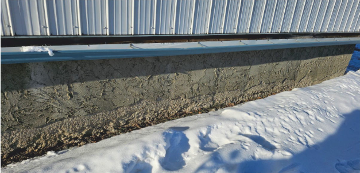
Photo 4. Exterior foundation erosion – East side
