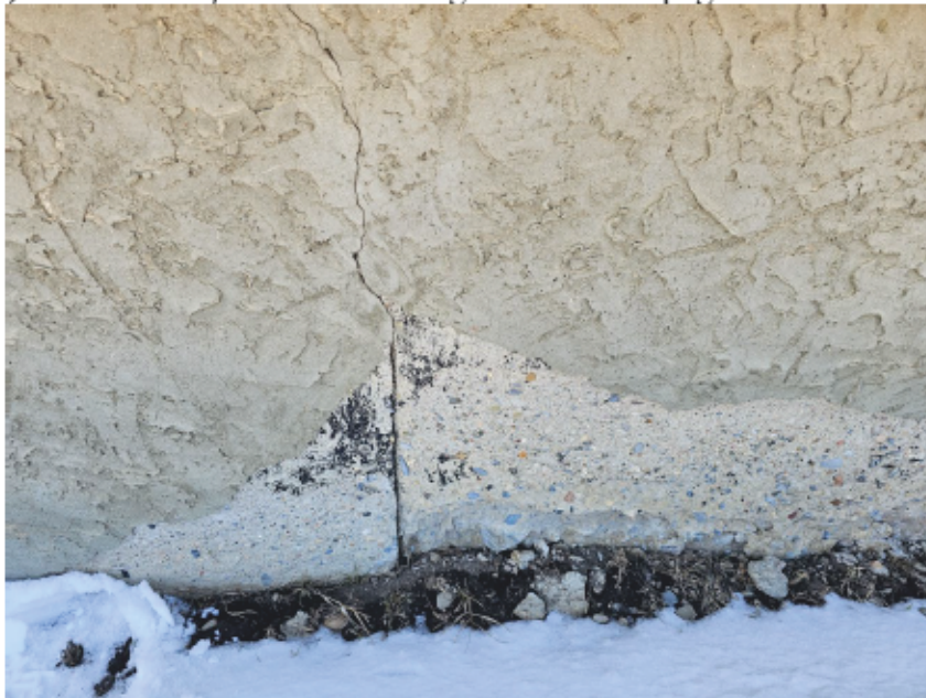
Photo 5. Foundation Cold Joints. – East side
