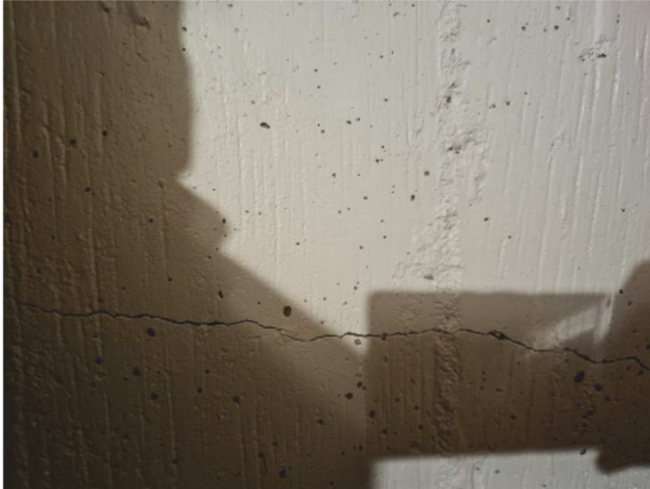
Photo 2. Interior View of Foundation Crack
