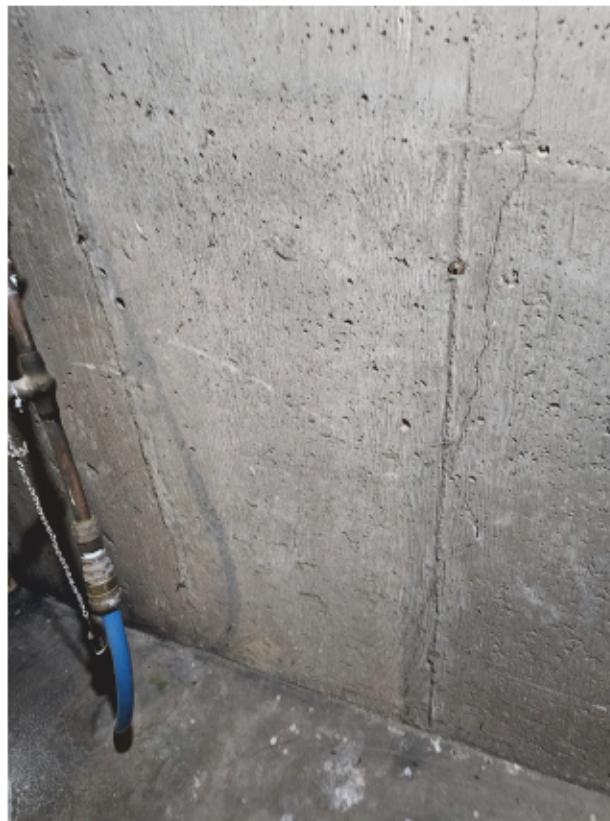
Photo 3. Interior View of Foundation Crack
