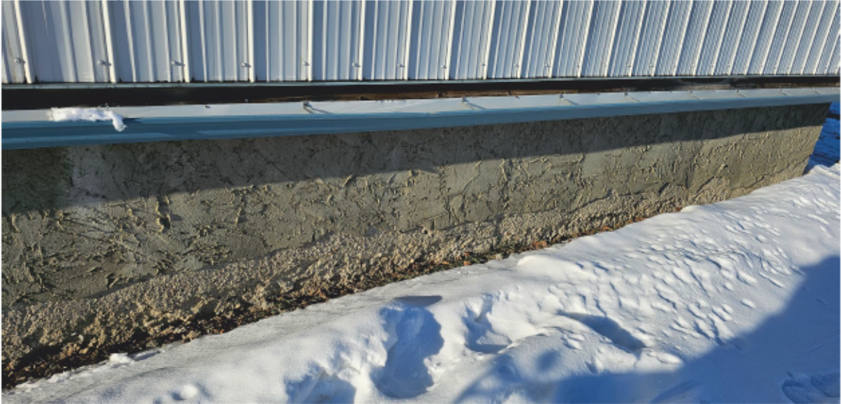
Photo 4. Exterior foundation erosion – East side
