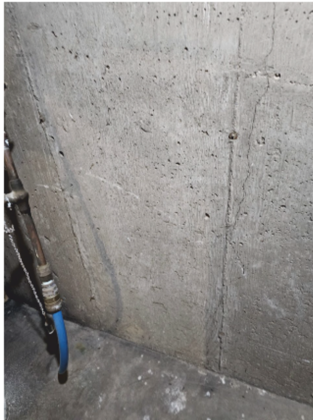
Photo 3. Interior View of Foundation Crack
