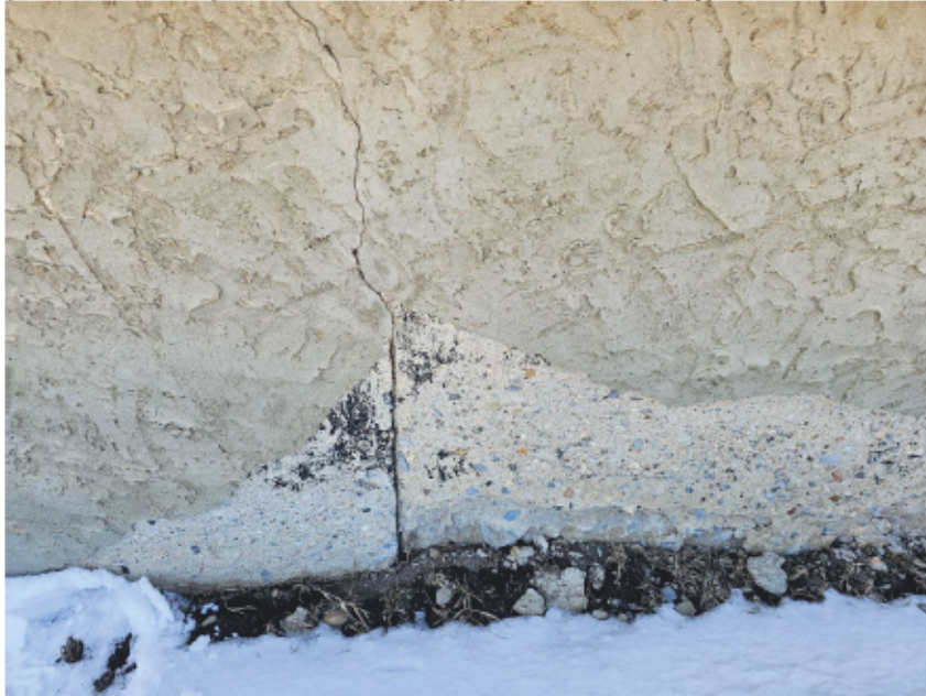
Photo 5. Foundation Cold Joints. – East side
