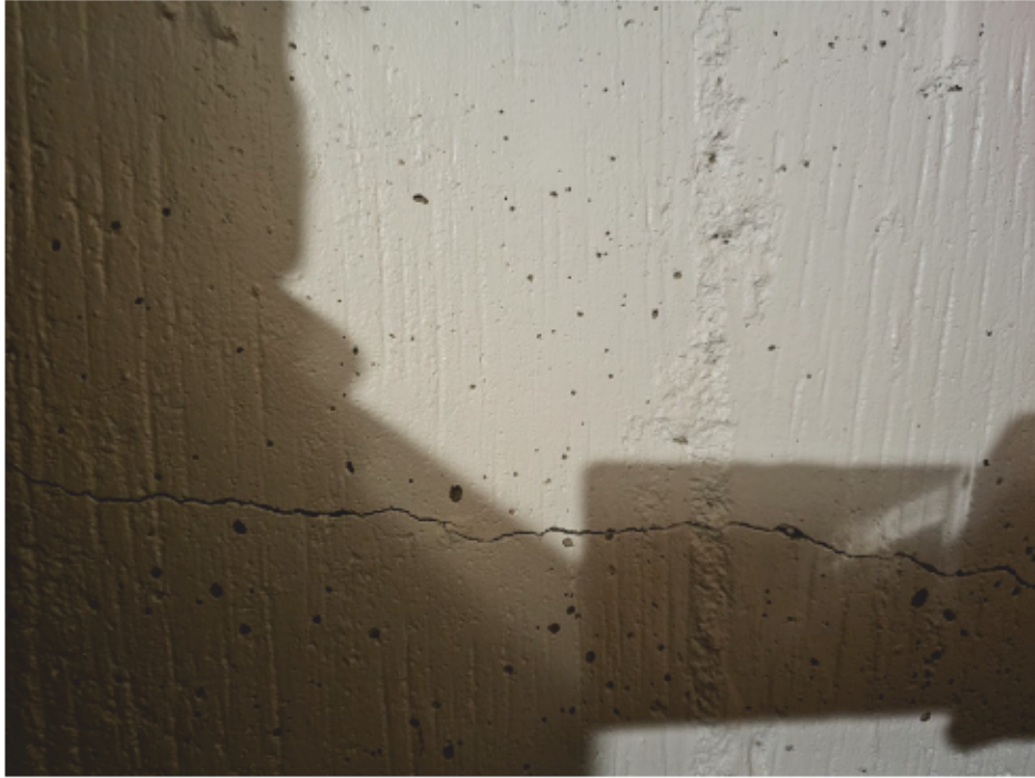
Photo 2. Interior View of Foundation Crack
