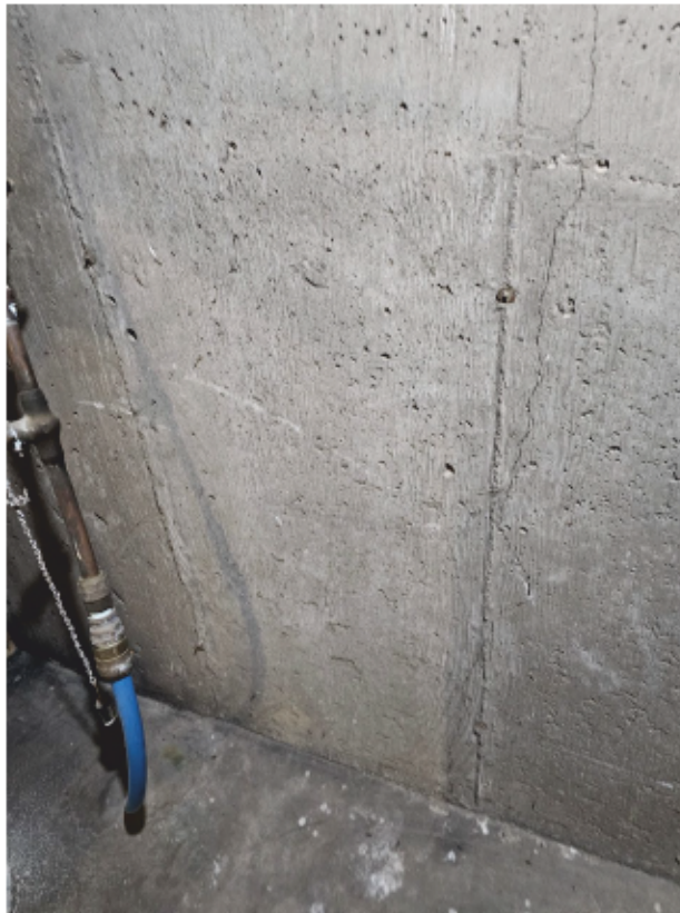
Photo 3. Interior View of Foundation Crack
