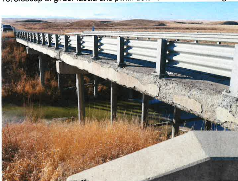
14. Close up of girder fascia and plinth deterioration undermining bridge posts.
