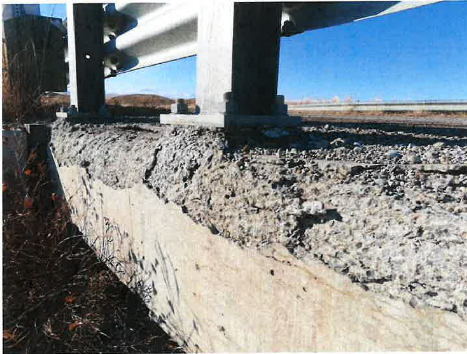
13. Closeup of girder fascia and plinth deterioration undermining bridge posts.
