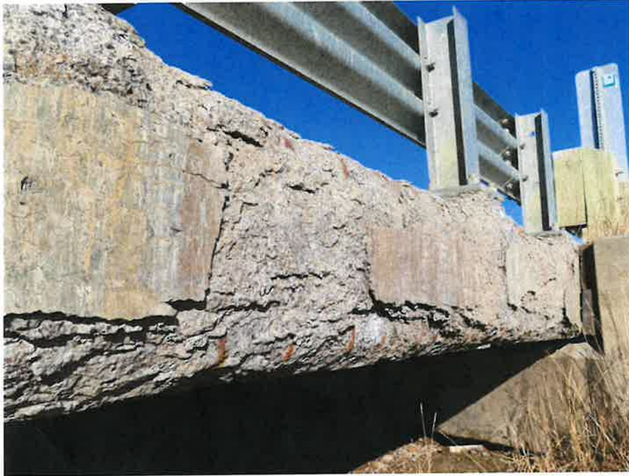
15. Close up of girder fascia deterioration with visible rebar stirrups and undermining posts.
